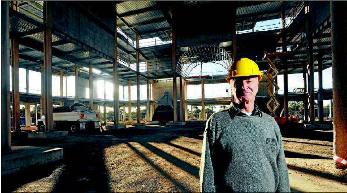
WORK IN PROGRESS: Ian Green on the site of the Great Stupa in Myers Flat. The stupa will measure 50 metres wide and 50 meters high
